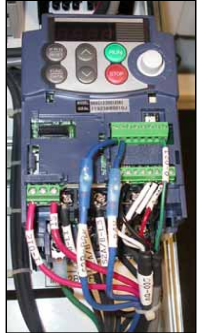
Figure 2: New 2hp VFD on a Cyber A/T Saw
